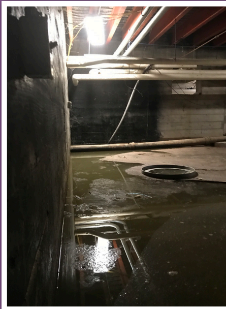
Shown above, water is pooled up in the basement and resting directly on the foundation of the building.
