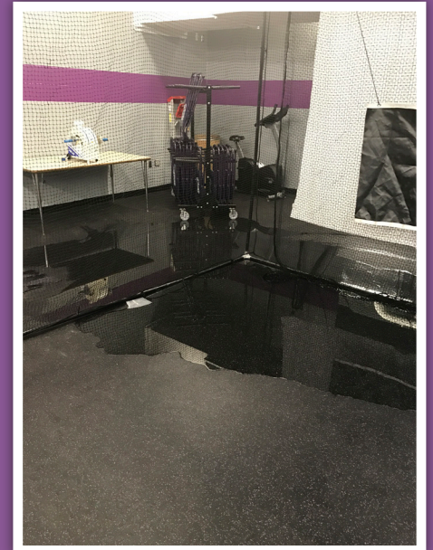
Flooding at Union Springs MS/HS isn't just experienced in the basement. As shown, these issues are felt in areas that students utilize on a daily basis.
